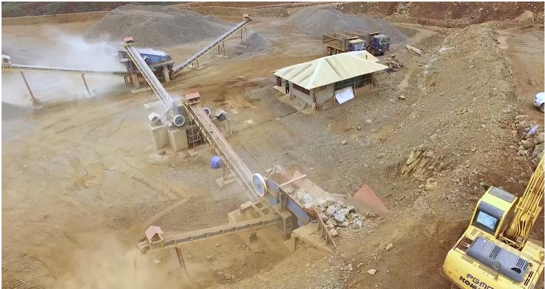
Figure 137. Aggregate Crushing Plant
